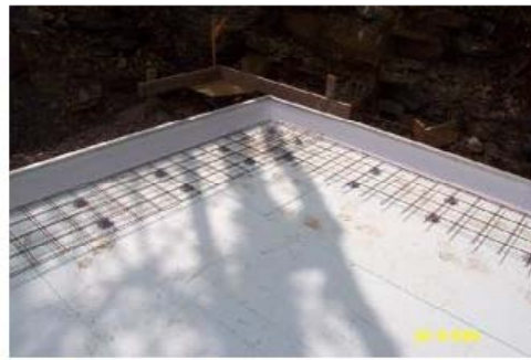
6. Install the bottom layers of wire mesh on chairs as per drawings (perimeter or bearing walls only)
