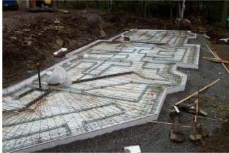
11. Install the top layer of wire mesh, and other rebar as per drawings
